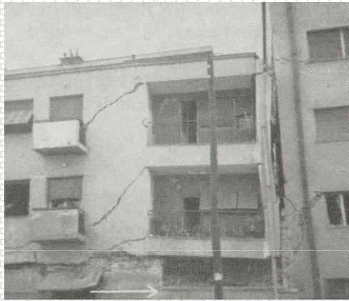
Failure owing to earthquake
